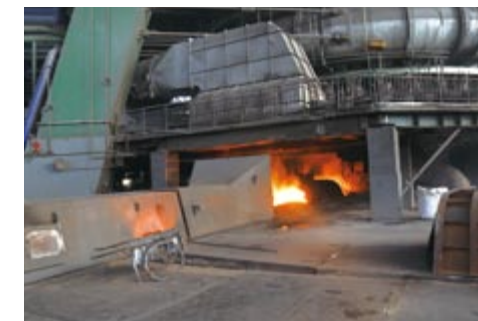
首钢京唐1#高炉出铁口的除尘效果 Dedusting effect at taphole of 1# BF, Shougang Jingtang
