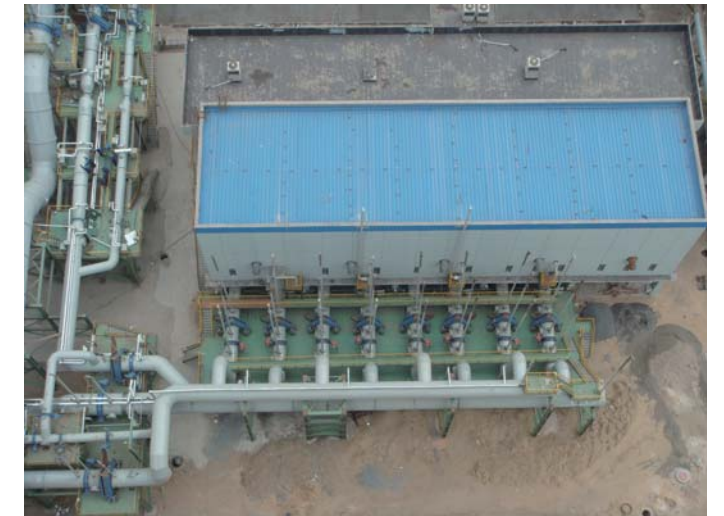
首钢迁钢转炉煤气加压站 Converter gas booster station in Shougang Qiangang
