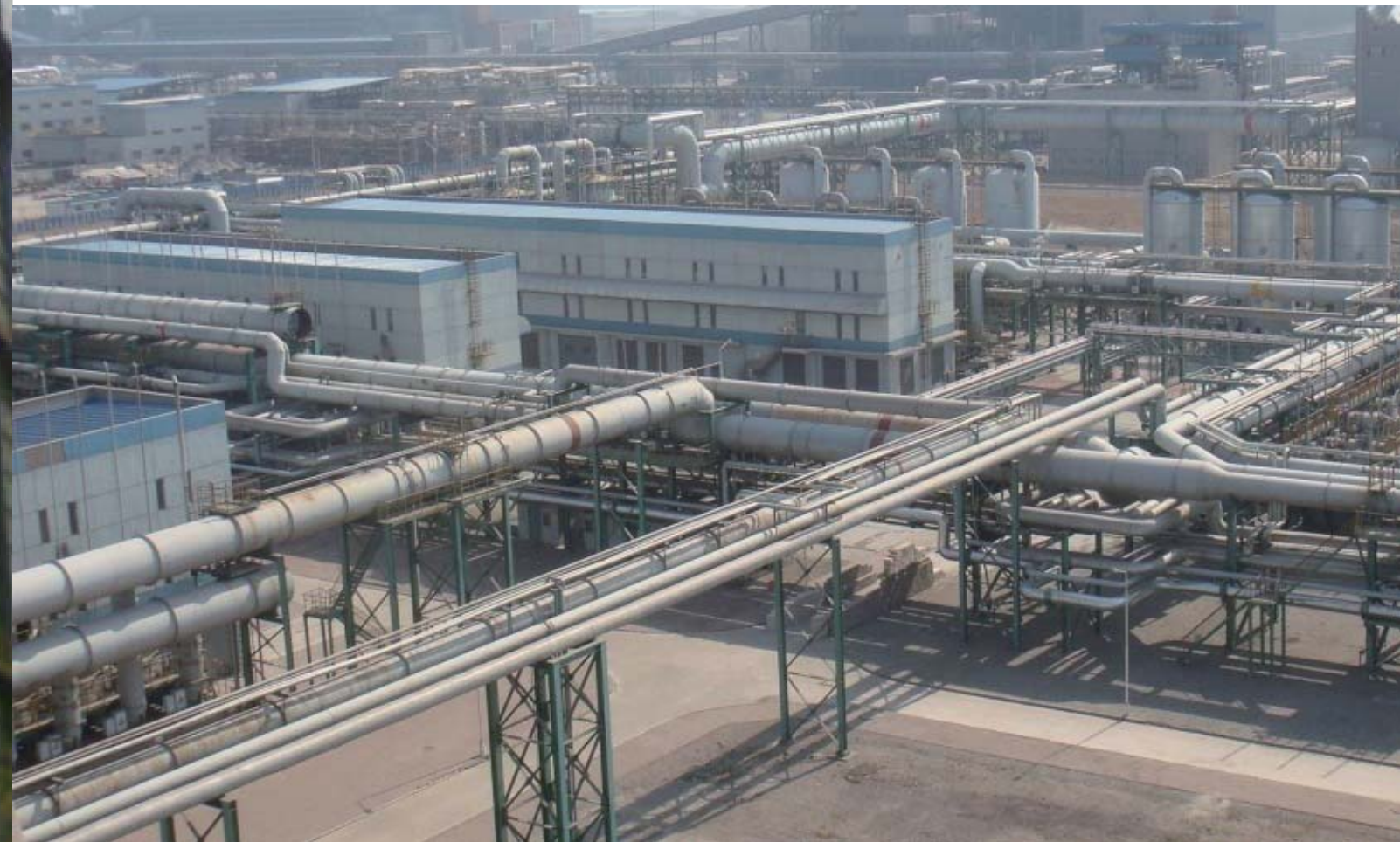
首钢京唐煤气储配站燃气设施 Fuel gas devices of gas storage and distribution station in Shougang Jingtang
