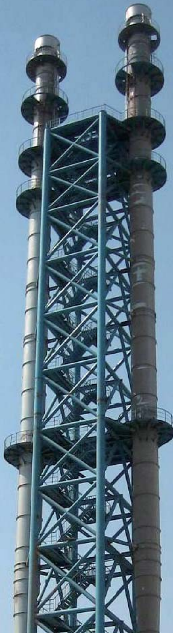
转炉煤气干法除尘煤气放散塔 Dry dedusting bleeder tower for converter gas
