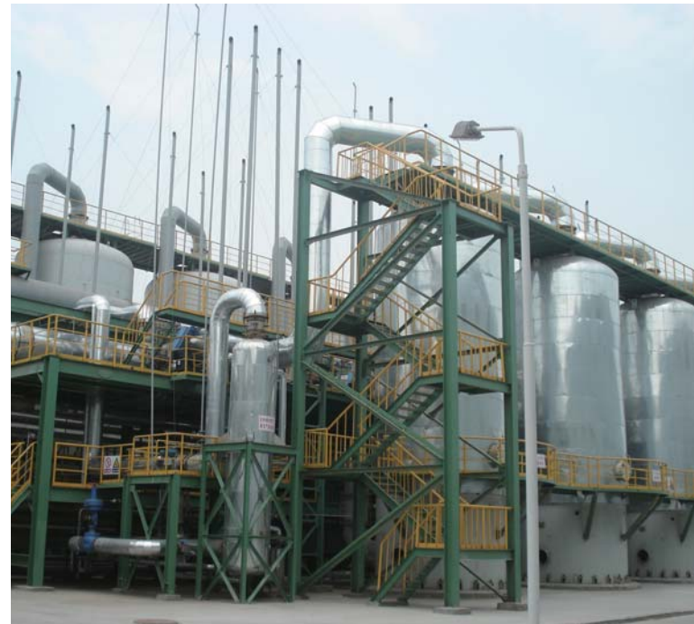
焦炉煤气二次净化系统（脱萘侧） Secondary purification system of coke oven gas (side of denaphthalene)
