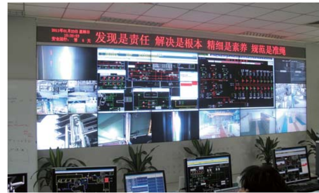
迁钢CCPP主控室 Qiangang CCPP main control room
