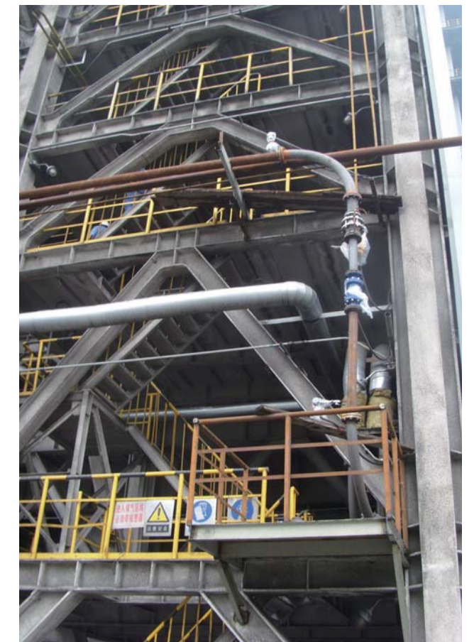
喷煤总管流量计和调节阀， 在线监测瞬时流量，控制喷煤量的瞬时波动 PCI main flowmeter and regulating valve for on-line monitoring instantaneous flow, controlling the momentary fluctuation of injection
