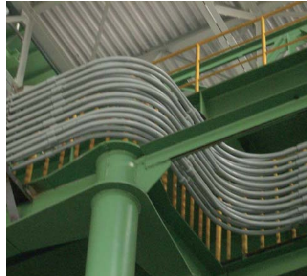
喷煤支管均匀布置 PCI branched pipes arranged uniformly
