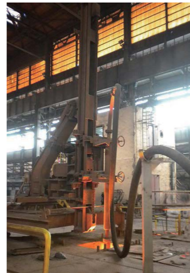
铁水“三脱”喷吹设施 “Desulphurization, desiliconization and dephosphorization” injection equipment for hot metal
