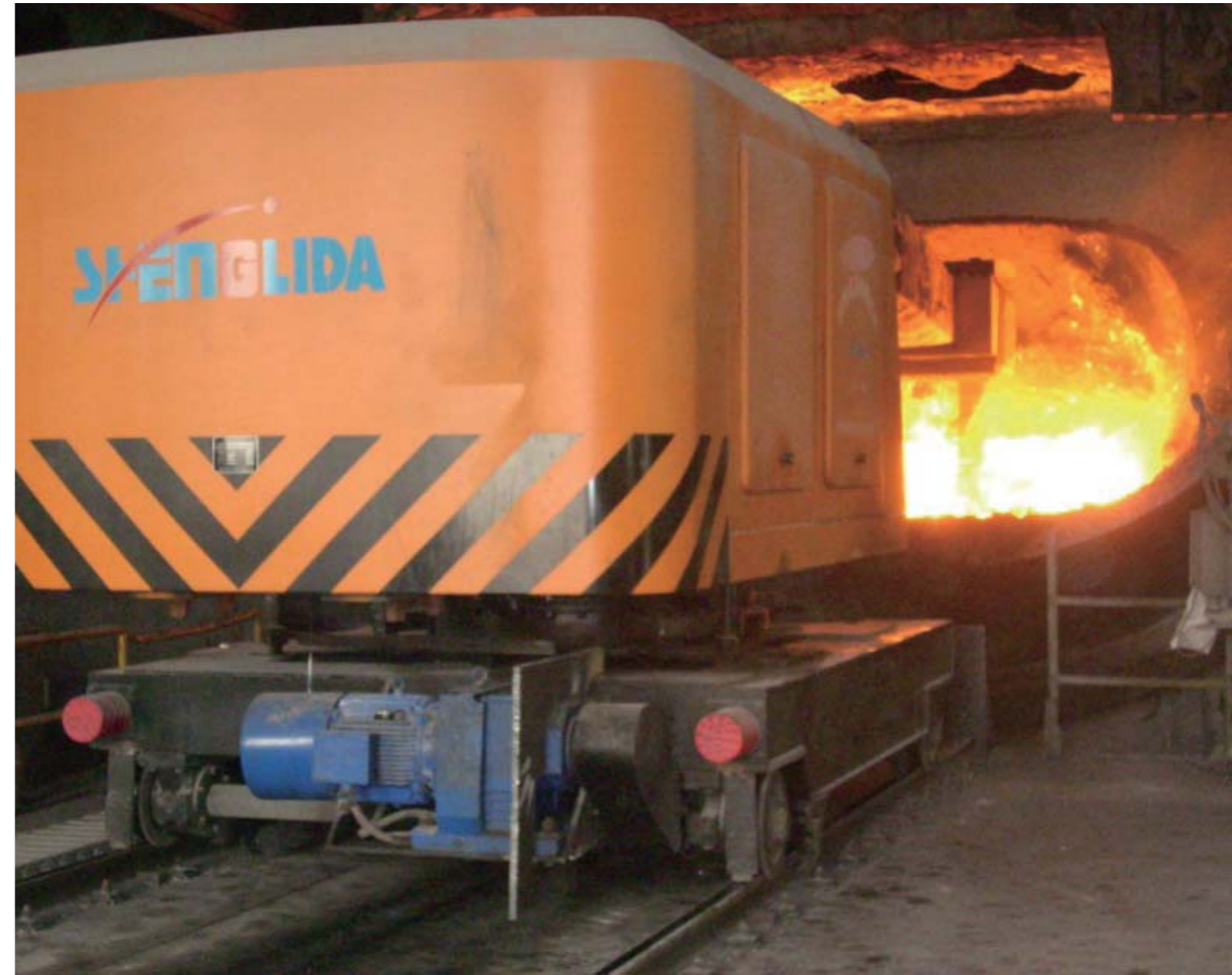
首钢京唐 KR 脱硫捞渣设施 KR desulphurization and slag skimming facility in Shougang Jingtang
