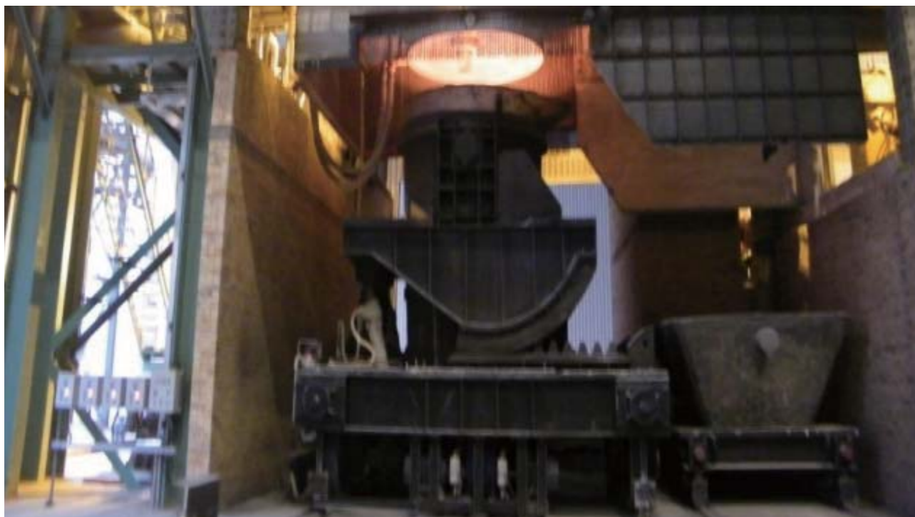
邢钢喷吹脱磷设施 Injection dephosphorization facility of Xinggang
